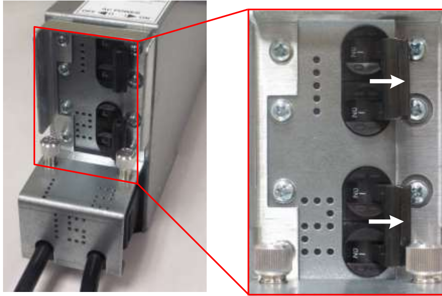
Figure 10-6 Power switches in the on position
