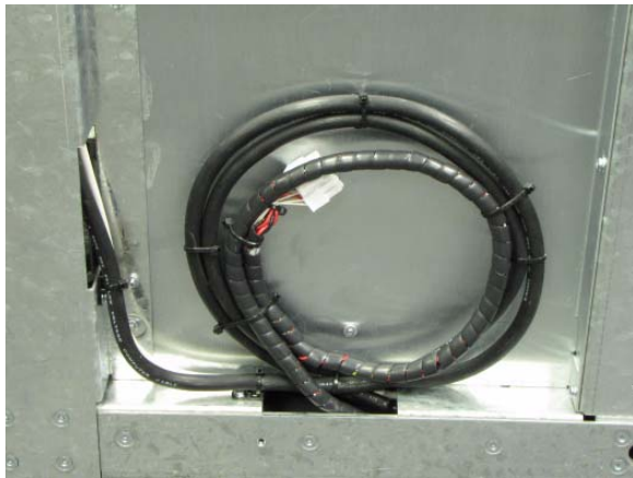
Figure 6-3 Expansion-pod controller cable on the side of the LRM
